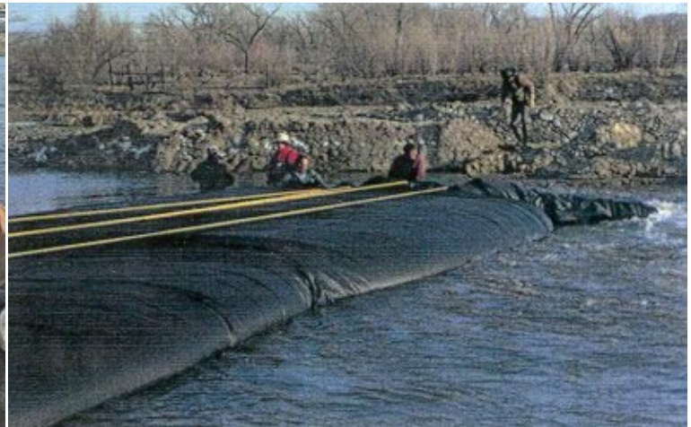
4. Unroll and fill... unroll and fill... unroll and fill... keeping continuous head inside.
