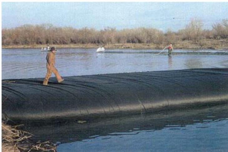
5. San Juan River. Main channel is completely blocked off.
